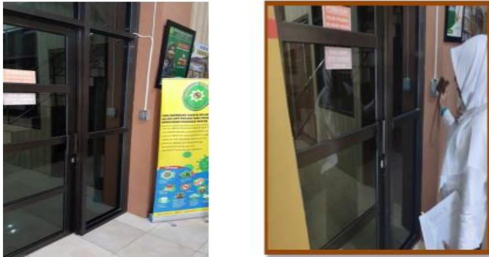
Gambar 5.3 : Door Lock System Pengadilan Negeri Tais
